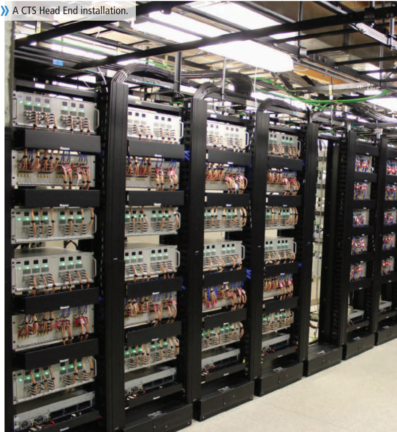
A CTS Radio Head installation. <<
